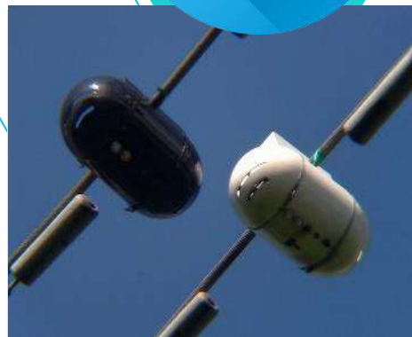
Dynamic Thermal Rating Monitoring
